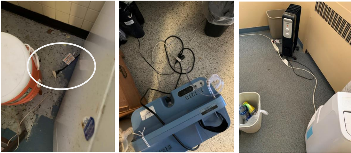
Photograph 17 (left): Kitchen refrigerator plugged into extension cord.
