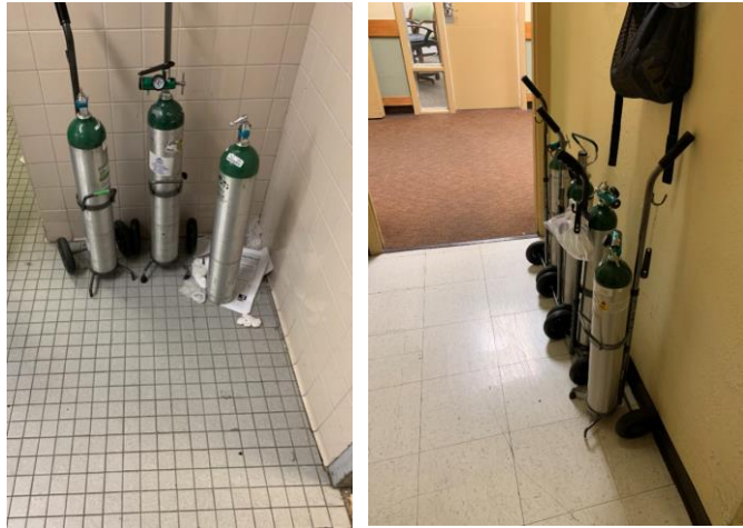
Photograph 12 (left): Improperly stored oxygen cylinders (in washroom). Photograph 13 (center): Improperly stored oxygen cylinders (in hallway).
