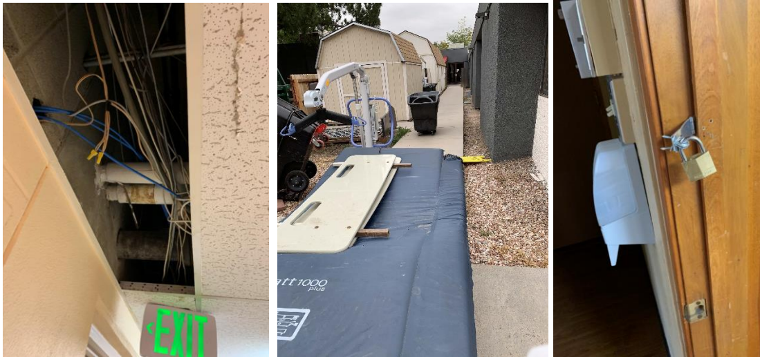
Photograph 1 (left): Missing ceiling tiles. Photograph 2 (center): Path of exit blocked. Photograph 3 (right): Padlock on patient room door.
